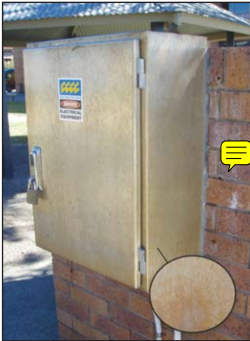
Figure 2 Tea staining is actually caused by salt building up in the crevices on the metal surface. This effectively concentrates corrosive chlorides in small areas, which can then be seen this corrosion.
